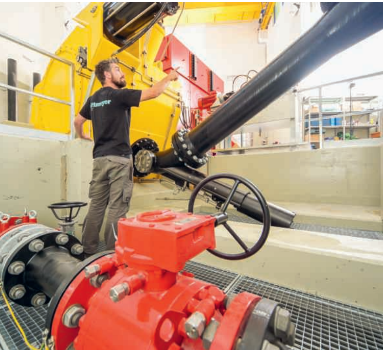
EW Mels power station Plons (SG)
