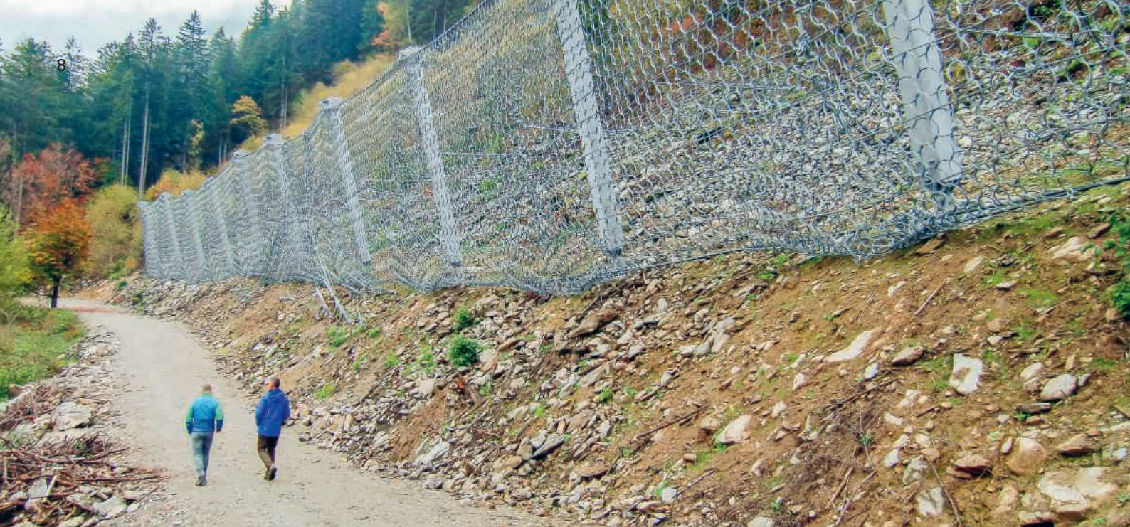
Pioneer: First 10,000 kJ rockfall protection barrier worldwide from Geobrug in Danielsberg, Austria
